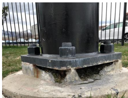
Figure 1. Poorly installed dry-packed grout pad
